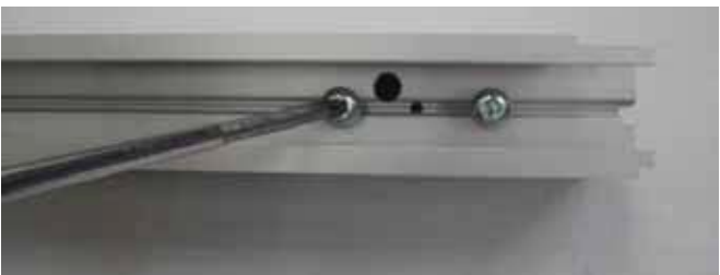
6.3 Insert detail [1] into the PAM45M profiles 3800 and 3813 or else the PAM45L profiles 3599 and 3822, and fasten it as shown in the diagram.
