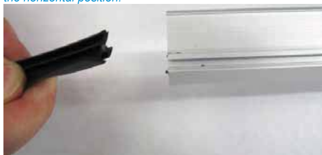
6.27 With PAM45M profiles, insert the seals into the glass-blocking profiles [8], as shown in the diagram.
