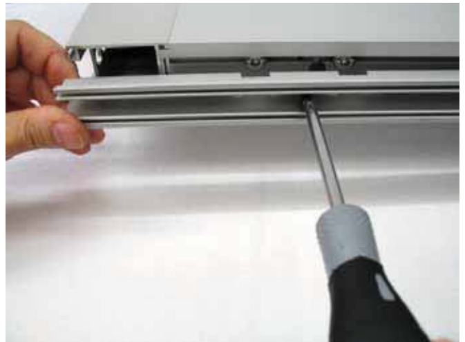
4.5 Fasten profile 3805 to the lower portion of the wing, as shown in the diagram.
