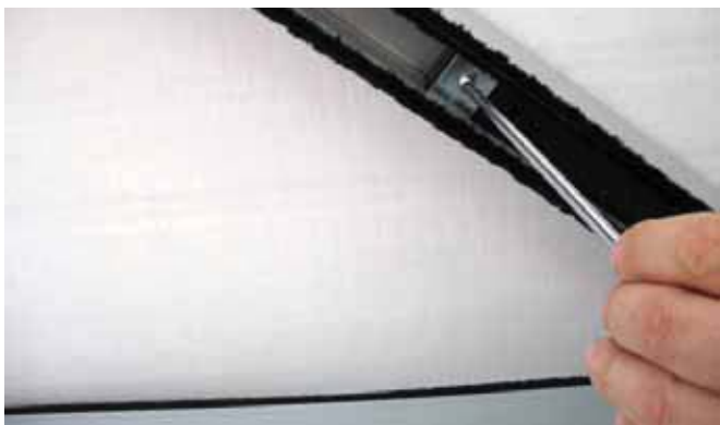
Note: during the installation of the fixture, in order to obtain the proper horizontal position of the mobile panic wing, loosen the fastening screws and adjust the screw shown in detail [3], as shown in the diagram.
